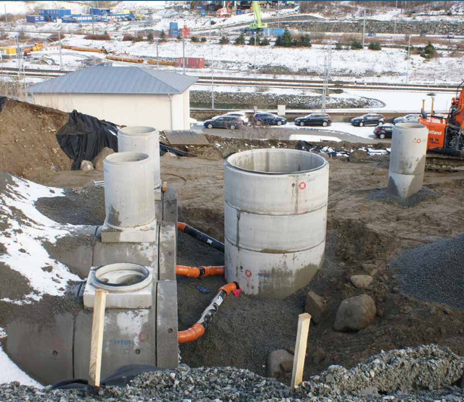
On the site of Multiblokk (Skjæveland Gruppen) south of Sandnes, the Norwegian Public Roads Administration has a pilot project to document the treatment efficiency, operation and maintenance of an implemented solution for treatment of stormwater from the new bridge and a connecting road.
