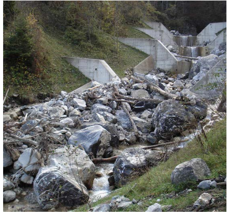
Debris flow passing check dam in Steinibach, Switzerland (Source: National Platform for Natural Hazard, Swiss Confederation)
