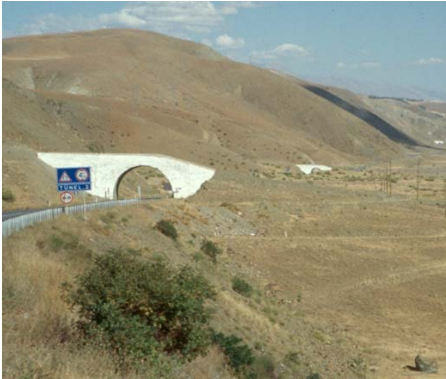
Bridges in eastern Turkey to allow debris flows from steep tributary valleys crossing a national road (Source: the Earth Physics Institute, the University Paris Diderot)
