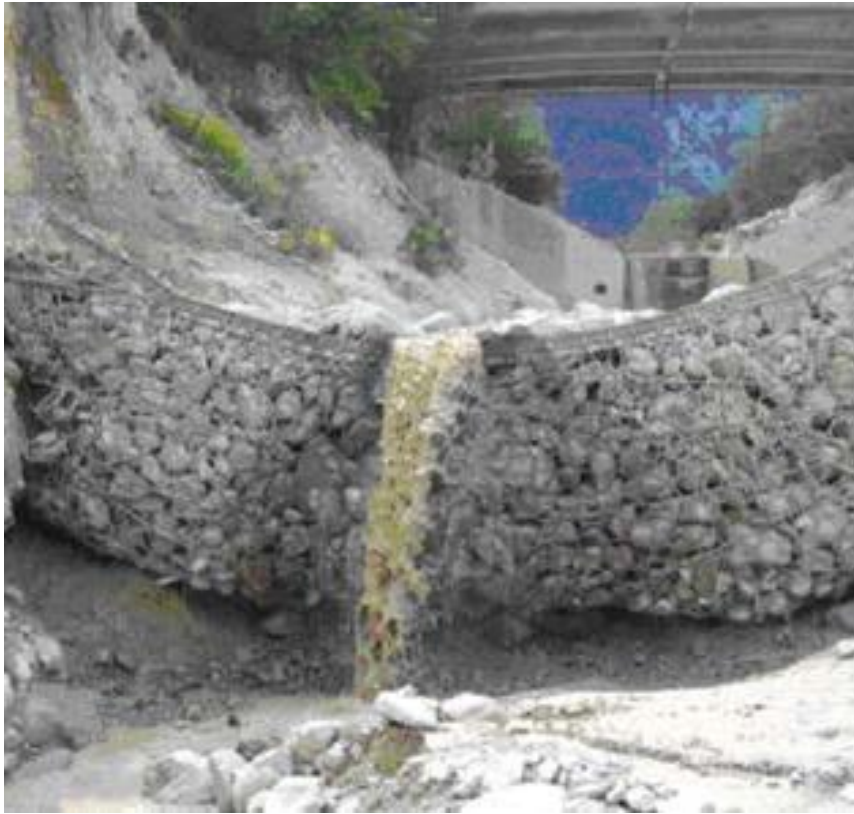
Flexible debris flow barrier (Source: WSL, Switzerland)
