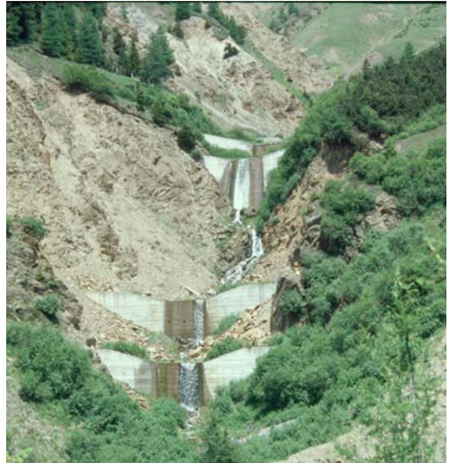
Check dams stabilizing a channel near Toblach, South Tirol, Italy (Source: the Earth Physics Institute, the University Paris Diderot)
