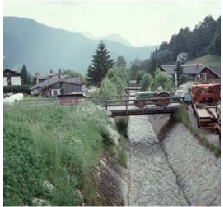
A shooting channel conducting a debris flow channel through the village of Matrei, Austria (Source: the Earth Physics Institute, the University Paris Diderot)
