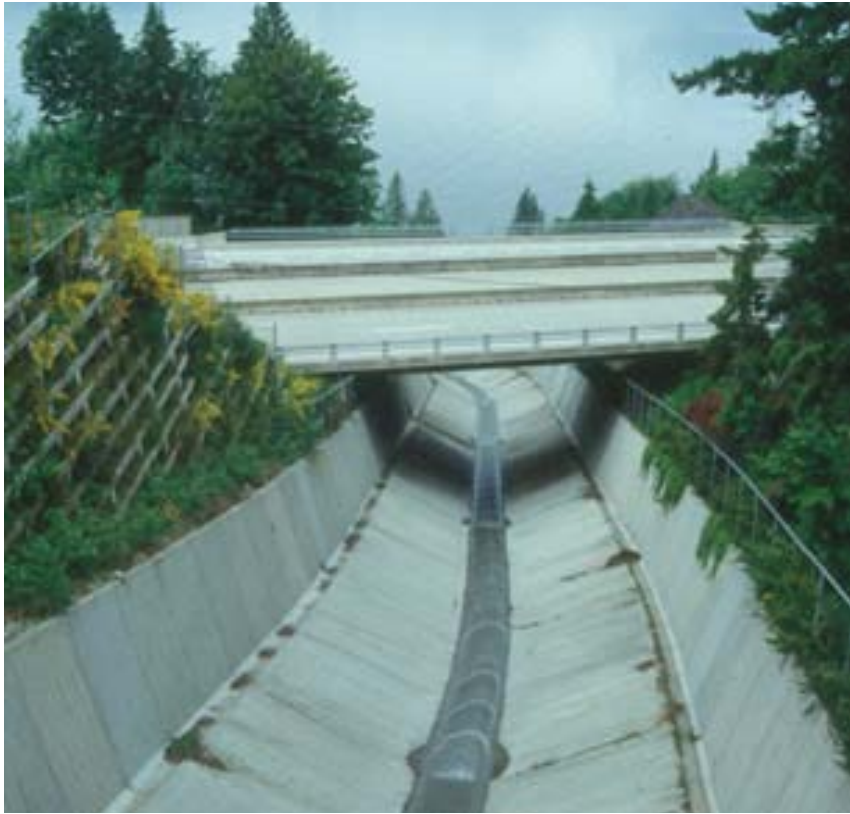
A lined channel designed for passage of debris flows on Alberta Creek, Lions' Bay, British Columbia (Source: the Earth Physics Institute, the University Paris Diderot)
