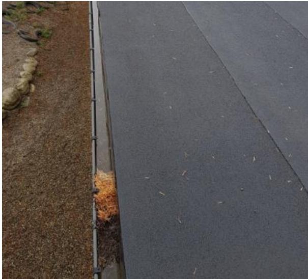
Pine needles clogging the roof drainage system.
