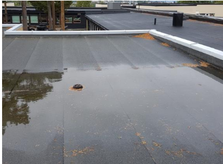
Pine needles clogging the roof drains.
