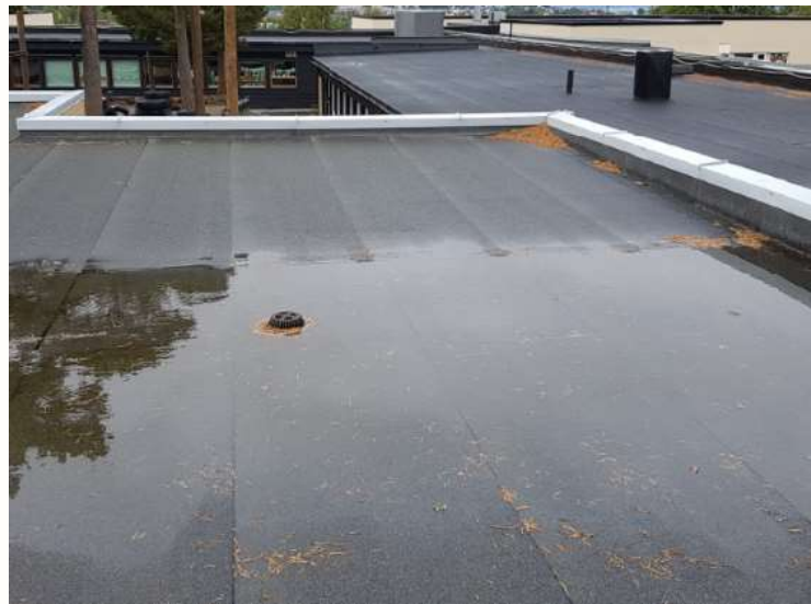
Pine needles clogging the roof drains.
