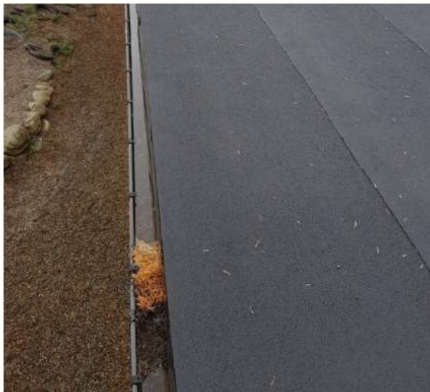
Pine needles clogging the roof drainage system.
