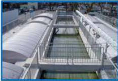
2. HOFFSELVA Local Treatment of Combined Sewer Overflows
