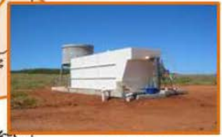
4. ATHENS AMI-Enabled Sewer Mining for water reuse
